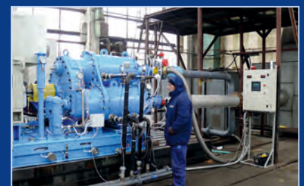
Centrifugal compressor skid.
