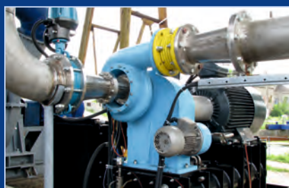
Centrifugal blower skid.
