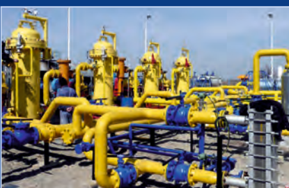
Screw compressor skids station.
